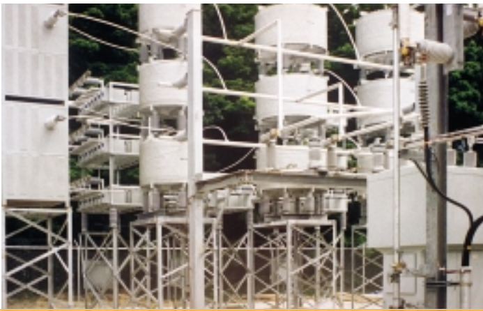
FILTER REACTORS SERVING AN INDUSTRIAL COMPLEX
